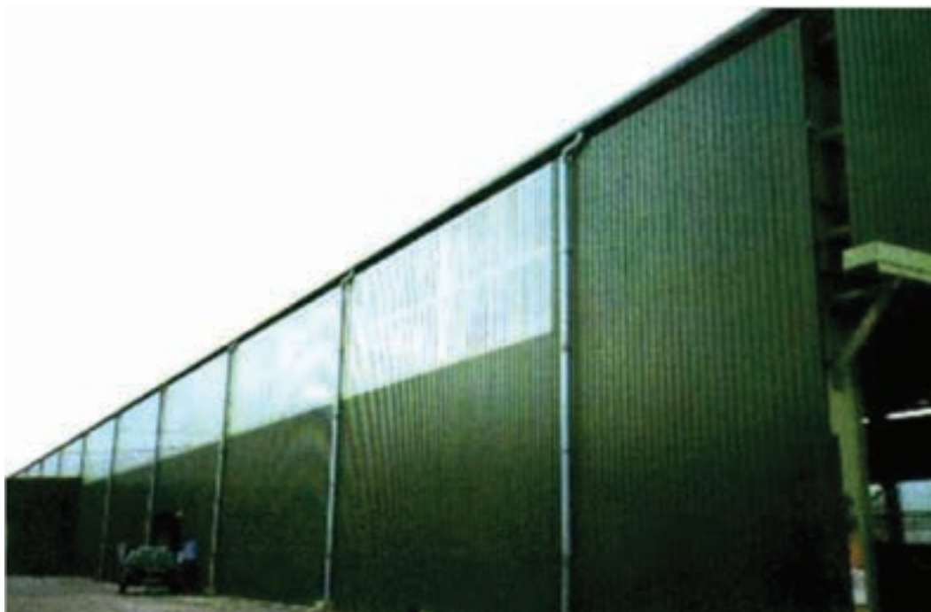
Figure 4.3: Lighting panels installed in the walls rather than the roof.
