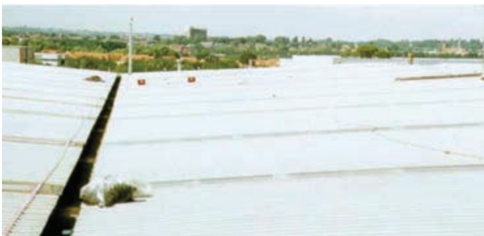
Figure 9.6: In some light conditions it is difficult to distinguish the rooflights from the metal sheets on this type of roof. Also the valley gutter is very narrow and rooflights extend down to gutter level. Both of these features increase the risk during cleaning maintenance and refurbishment.
