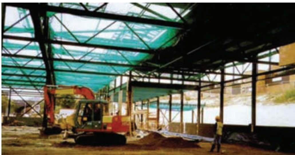
Figure 11.4: Debris netting in addition to safety netting may enable work to be carried out safely below roof workers
