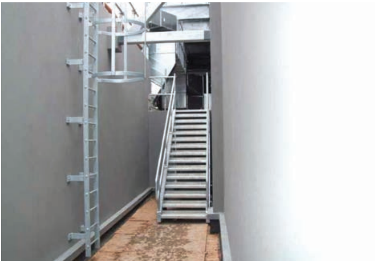
Figure 4.6: Examples of permanent access ladders and gantries.
