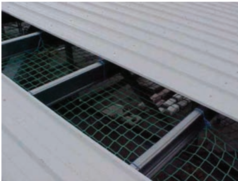
Figure 9.3: Industrial roofwork: Use of safety nets.
