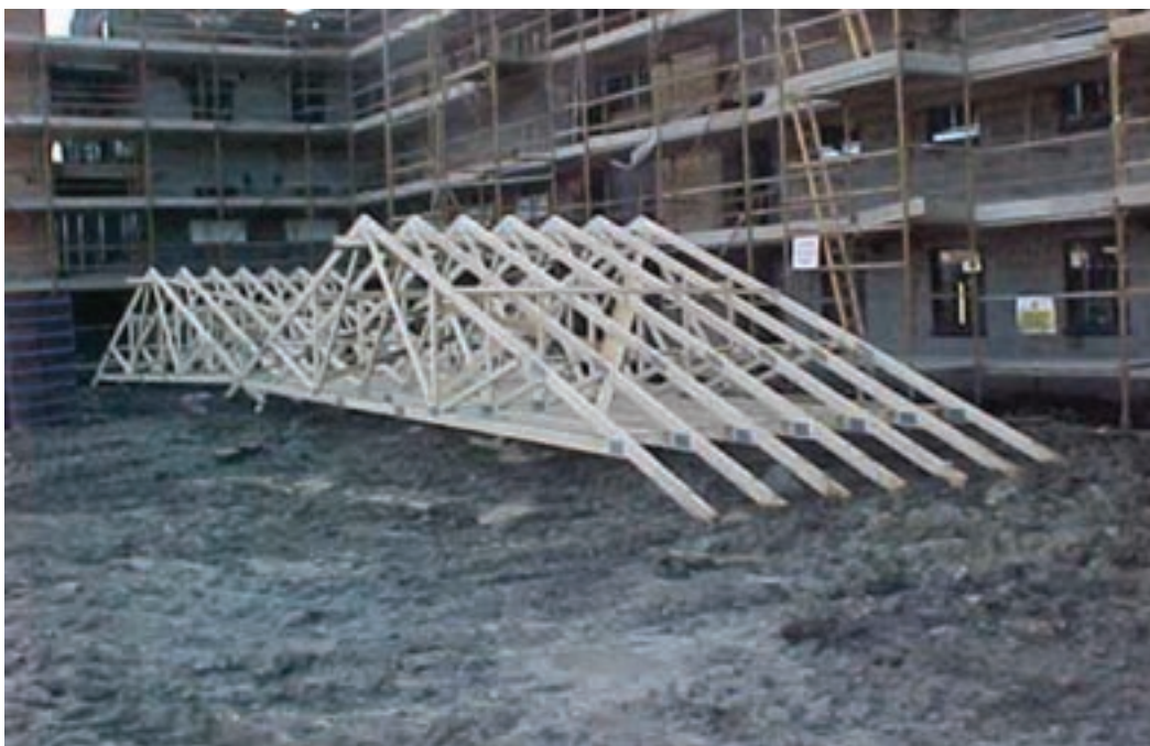
Figure 8.1: Lifting pre-assembled roof into position by crane greatly reduces the need for work at height.
