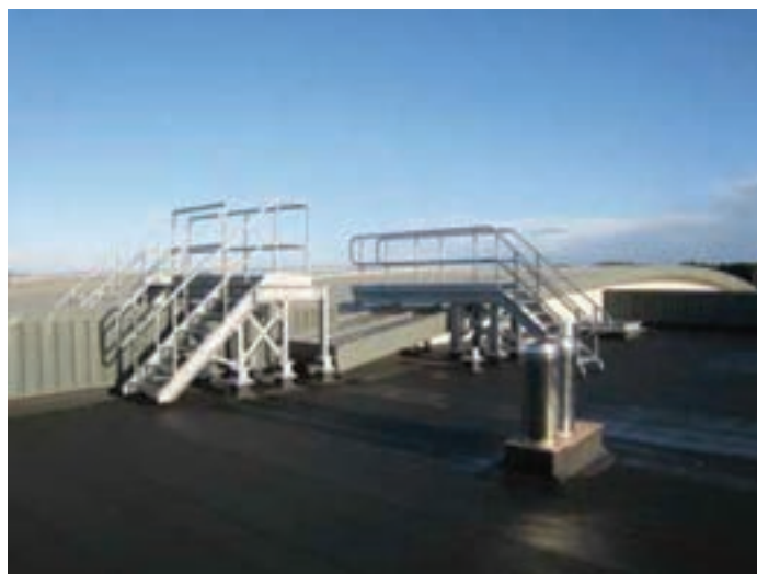
Figure 4.2: Permanent access stairs giving safe access to different roof levels. (This permanent stair access was included in the initial design).
