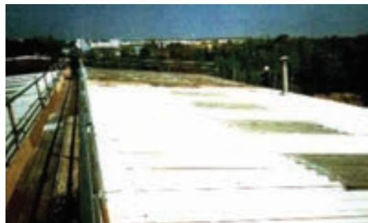
Figure 9.5: Cleaning a fibre cement roof using a self-contained water fed brush unit. There is no need for access onto the roof sheets and the guard-rails prevent workers falling onto them. (Note: waste water is filtered before disposal).
