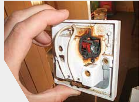
Potential ignition source from electrical equipment.
