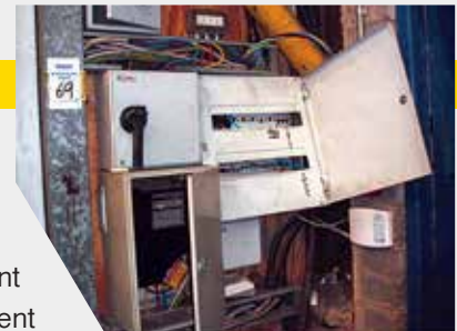
Installations like these can lead to inadvertent contact and electrocution.
